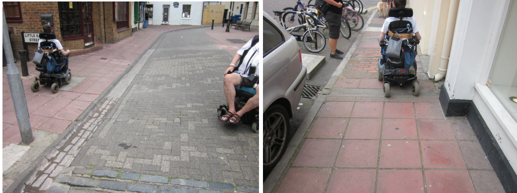
14. Little East Street. Drainage gully makes it hard for wheelchairs to cross.
