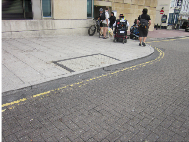
13. Kings Road near Thistle car park entrance. Tactile paving leads to a step. Dropped kerb required.
